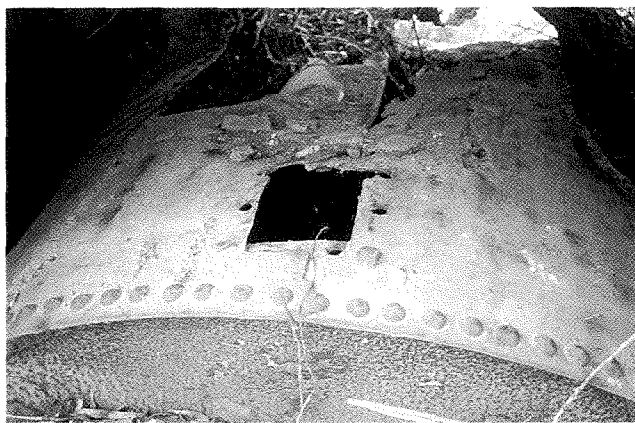
Fig. 6: The exit for the vaporised oil in the top of the retort. In this case the circular opening for the 10 cm pipe had been damaged and a repair was done by attaching a square plate which housed the pipe connection. There are many effective repairs to retorts done by the Joadja blacksmith. (R. Ian Jack 1996).
