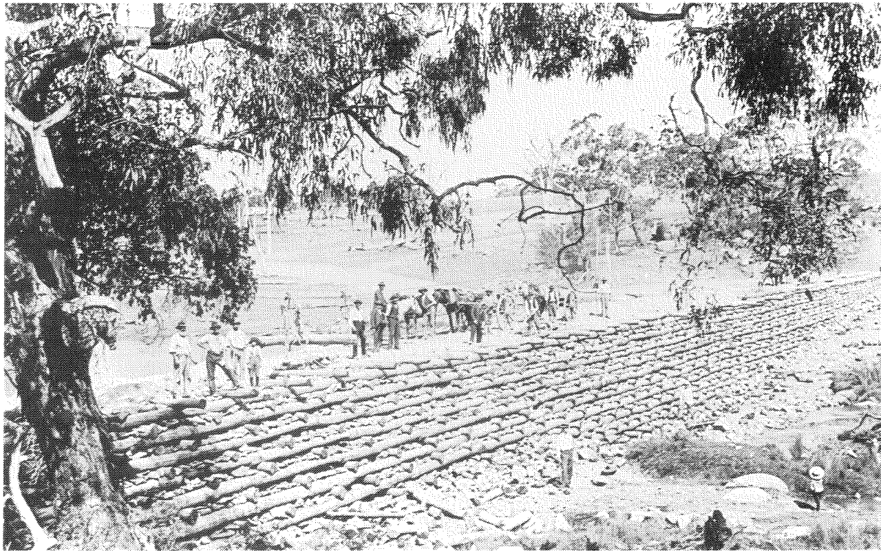
Fig. 5: Dam under construction across the Gara River at the Blue Hole. Undated. (University of New England Archives.)
