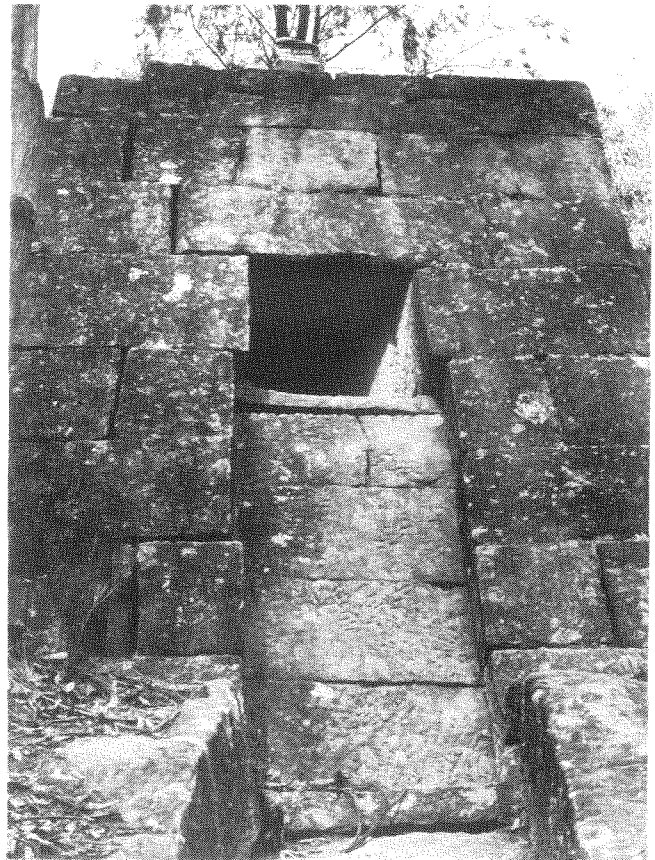
Fig. 9: Type 3b stonework on the first and most southerly of the four (originally five) buttresses on Devine's Hill, showing the mouth of the culvert with the race and part of the flume below. The work answers the description of ashlar masonry, with stones dressed to given dimensions (averaging 30×30–60×30cm), evenly coursed and tightly jointed. (Photograph by G. Karskens.)
